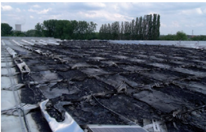
Area of roof after damaging event
