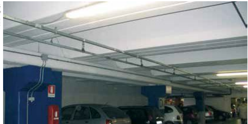
Canalis KBA supplying luminaires nearby sprinklers.
